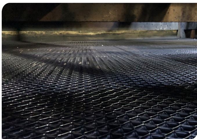
Brentwood's OF21MA is installed, delivering proven performance.
