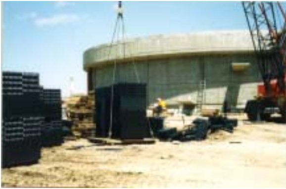
Wooden platform with wire cables
