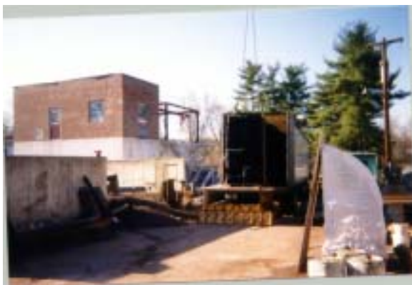
Media unloading platform
