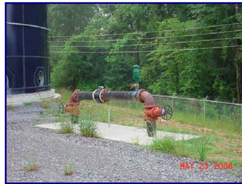
Figure 3 Filter influent meter
