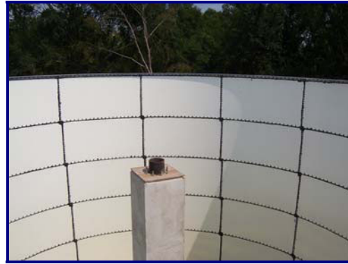
Figure 5 Stationery support pier for the distributor
