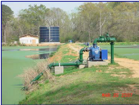
Figure 2 Filter influent pumps in Cell #3
