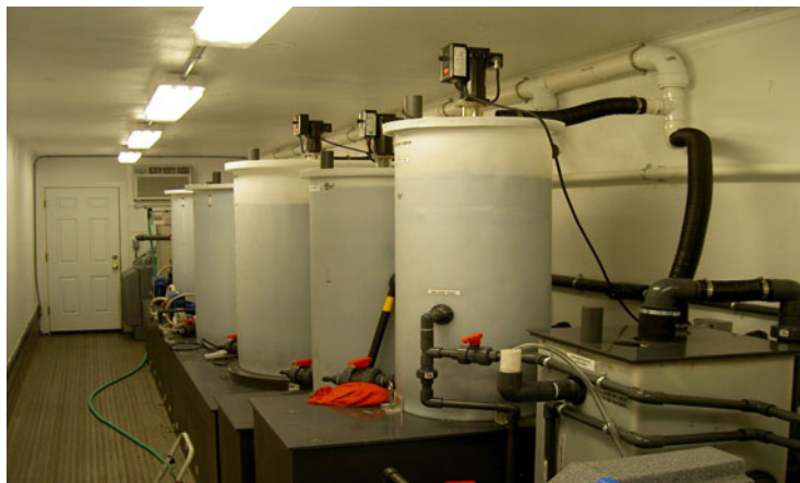
Figure 1 Interior photograph of the pilot trailer
